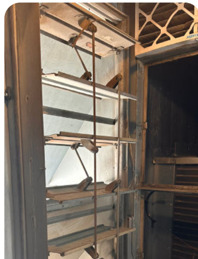
Rusted Actuators Failed Leading to Freeze
